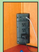
Corner mounted data/electric port with RJ-45 and CAT-5 wiring.
